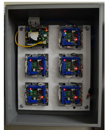
A. S. WISE custom-designed panel at personal care products manufacturing plant.
